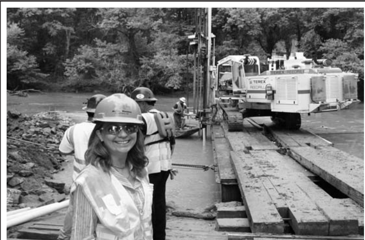
Have you seen something you think may impact or pollute our waterways? Call UCR's hotline at (404) 352-9828 ext.16 or go to www.chattahoochee.org and click on "Report a Problem." Above, UCR's General Counsel Juliet Cohen visits a construction site for a sewage outfall pipe in response to a hotline call.
